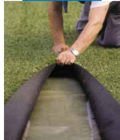
Installation of synthetic grass flooring with Adesilex G19 - S.Siro Stadium - Milan - Italy
